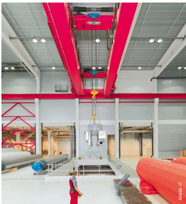
Load handling at two operating levels: Demag crane in stock preparation
